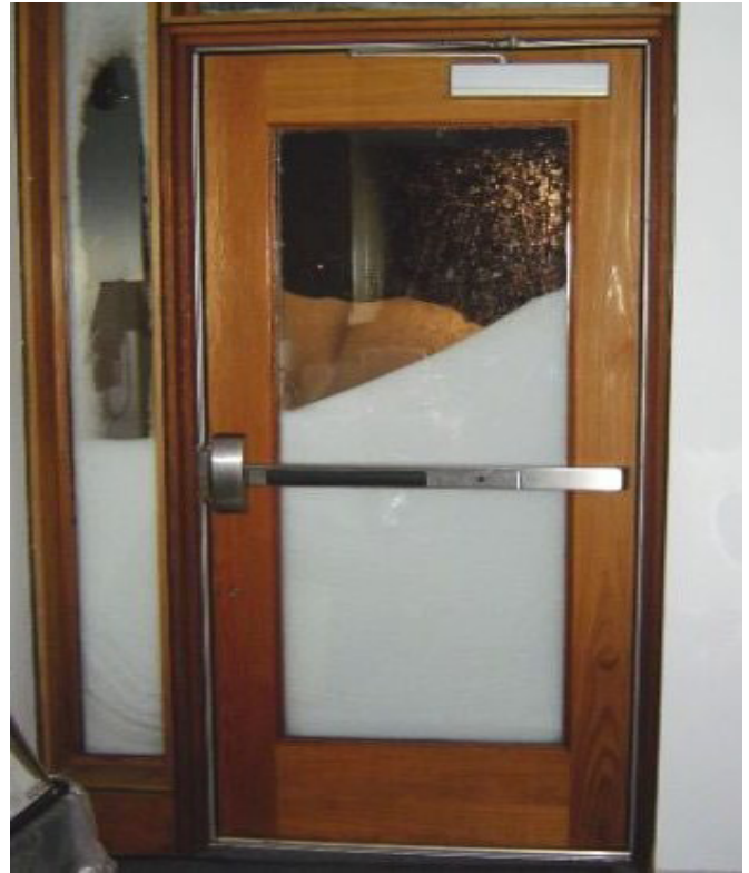
Snow buildup at an exit posing a fire hazard PHOTO: NOAA
