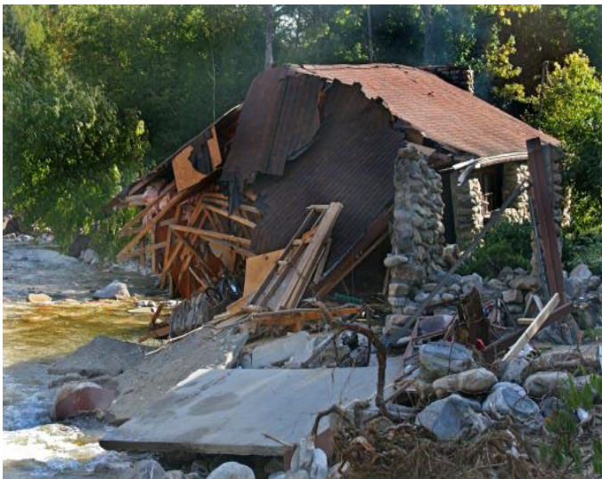
A Vermont house undercut during flooding caused by heavy rains following Tropical Storm Irene FEMA PHOTO
