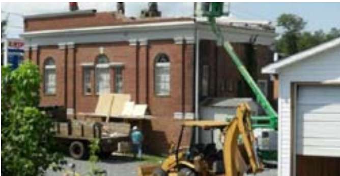
Earthquake Damage to the Mineral Virginia Town Hall being repaired. EERI PHOTO
