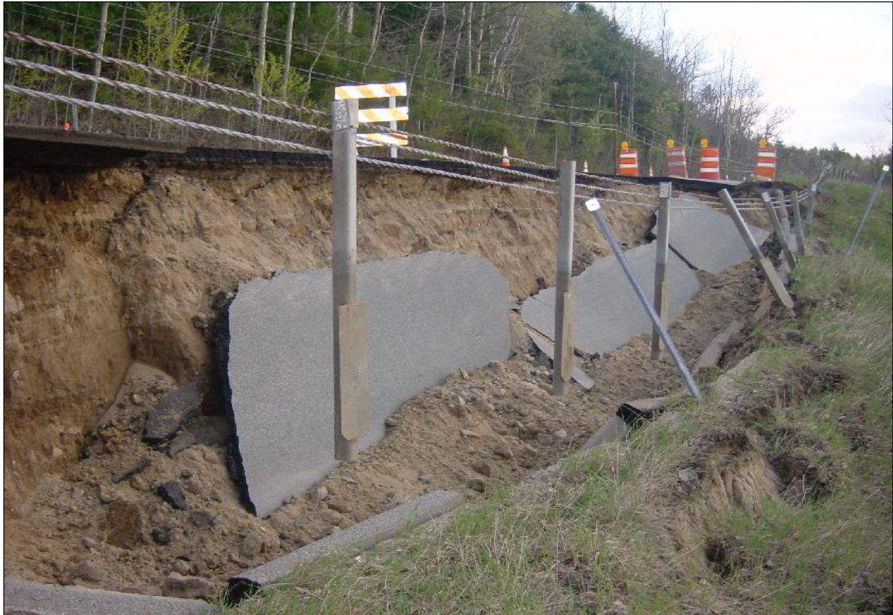
ROAD DAMAGE CAUSED BY THE AUSABLE FORKS, NY EARTHQUAKE OF APRIL 20, 2002
